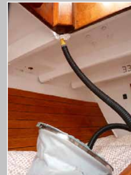
Your dinghy inflation pump can be used to trace the point of origin of deck leaks
