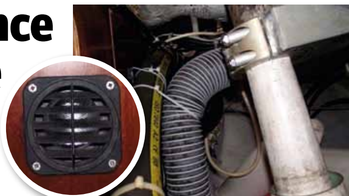
INSET The new heater inlet in the aft cabin bulkhead MAIN The sugar scoop looks tidier with new ducting and re-routed wiring
