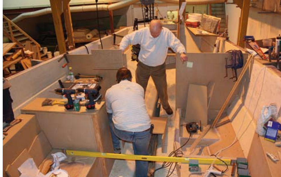
More bulkheads and the major structures of the interior come next, fitted to the lines marked inside the hull at the outset. Here the designer, David Thomas (right), and the interior plug-maker, Richard Dickson, look at the engine bed and the alignment of the prop shaft. Note the cooker in position in the galley
