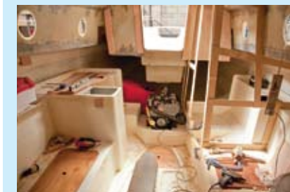
Another test-fit of the deck with the interior partly fitted out. Stick templates are made for the heads bulkheads
